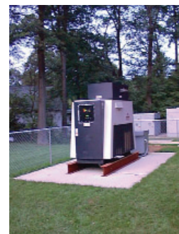
Front view of the microturbine installed at the Chesapeake Building
